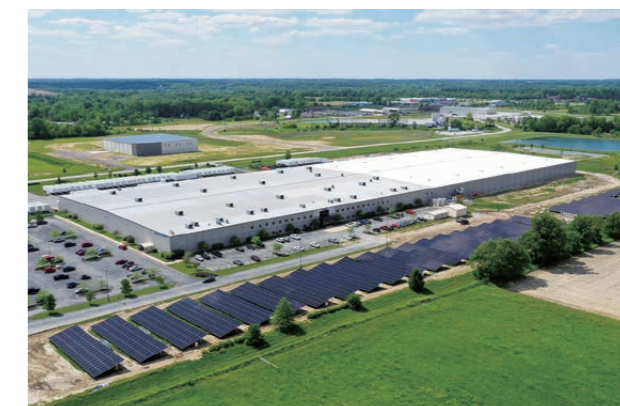
Newly installed solar power generation system at TS TECH INDIANA, LLC
